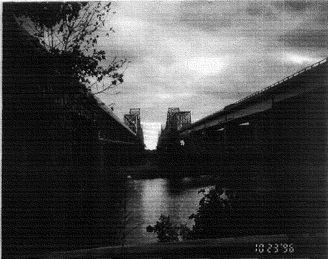
Figure E-3 The US 41 Northbound Approach Bridge at Evansville, IN (Northbound on left side in the picture)
