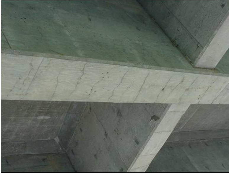
(a) Flexural crack in one of the girder
