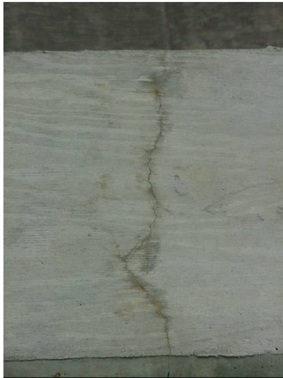
(b) Close-up of a flexural crack
