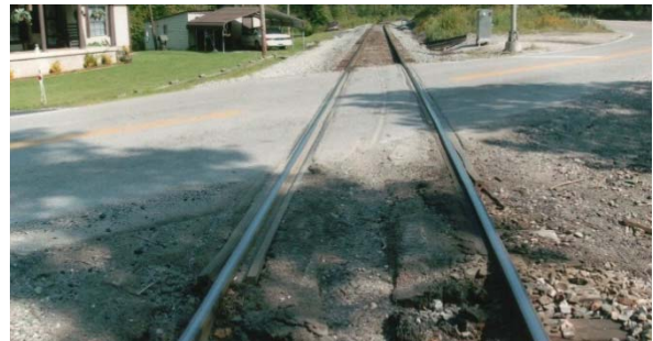
August 2009, Note Scar From Derailed Wheel
