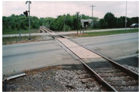
May, 2008, Slight Releveling of Asphalt Approaches
