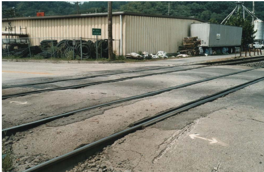
U.S. 60, 35 th Street in Catlettsburg in 2006 just prior to Renewal with Concrete Surfaces
