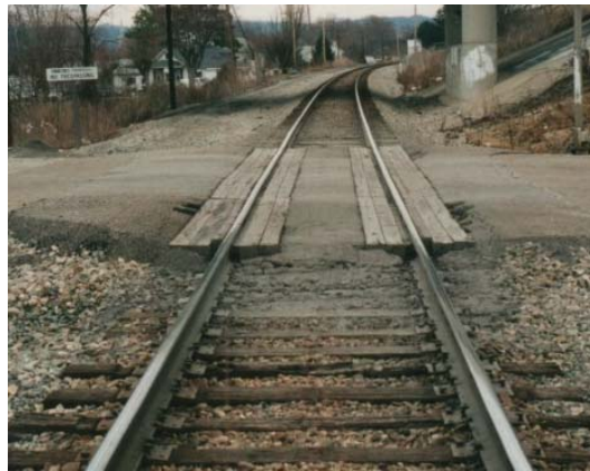
South Portsmouth Access Road in 2002 prior to Renewal with LT Resources Composite Surface
