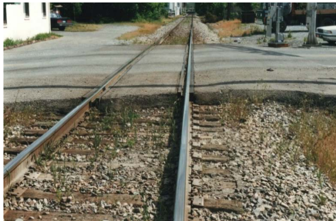
1999 Before Renewal, Note the Settlement and Roughness
