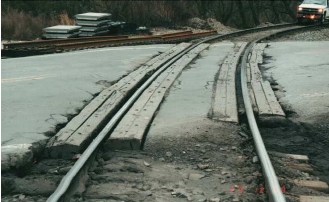
Figure 3.13. Settlement and surface deterioration.
