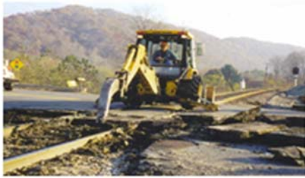
KY 3 Condition prior to rebuild
