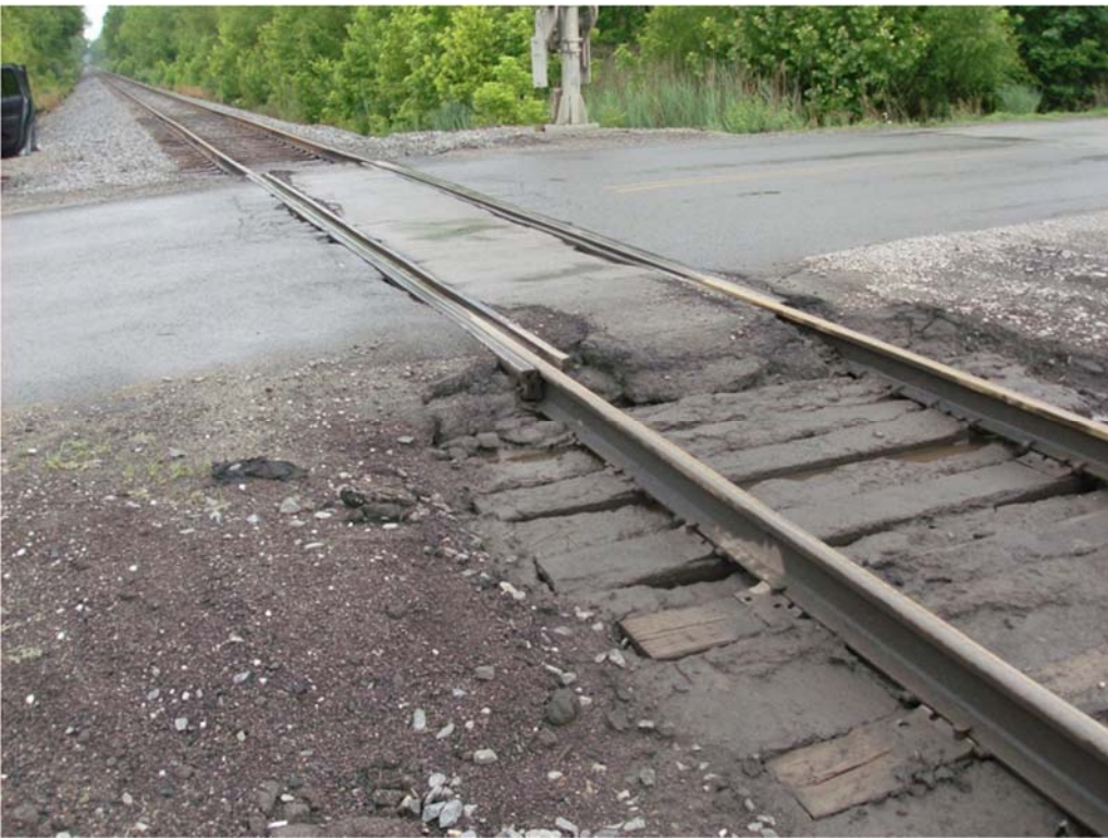
Figure 3.12. Settled and pumping crossing, lack of support.
