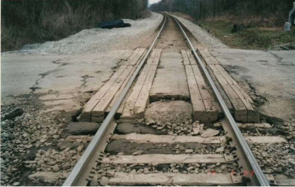
Figure 3.11. Poor quality support.
