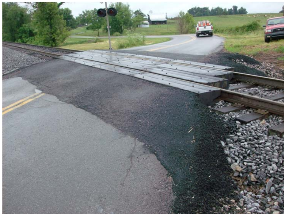
Figure 3.3. All Timber surface, approaches too short.
