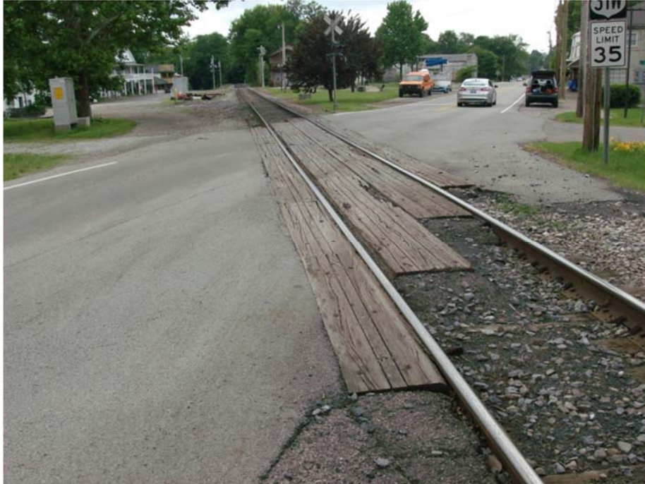
Figure 3.9. Deteriorated all timber crossing, still smooth.
