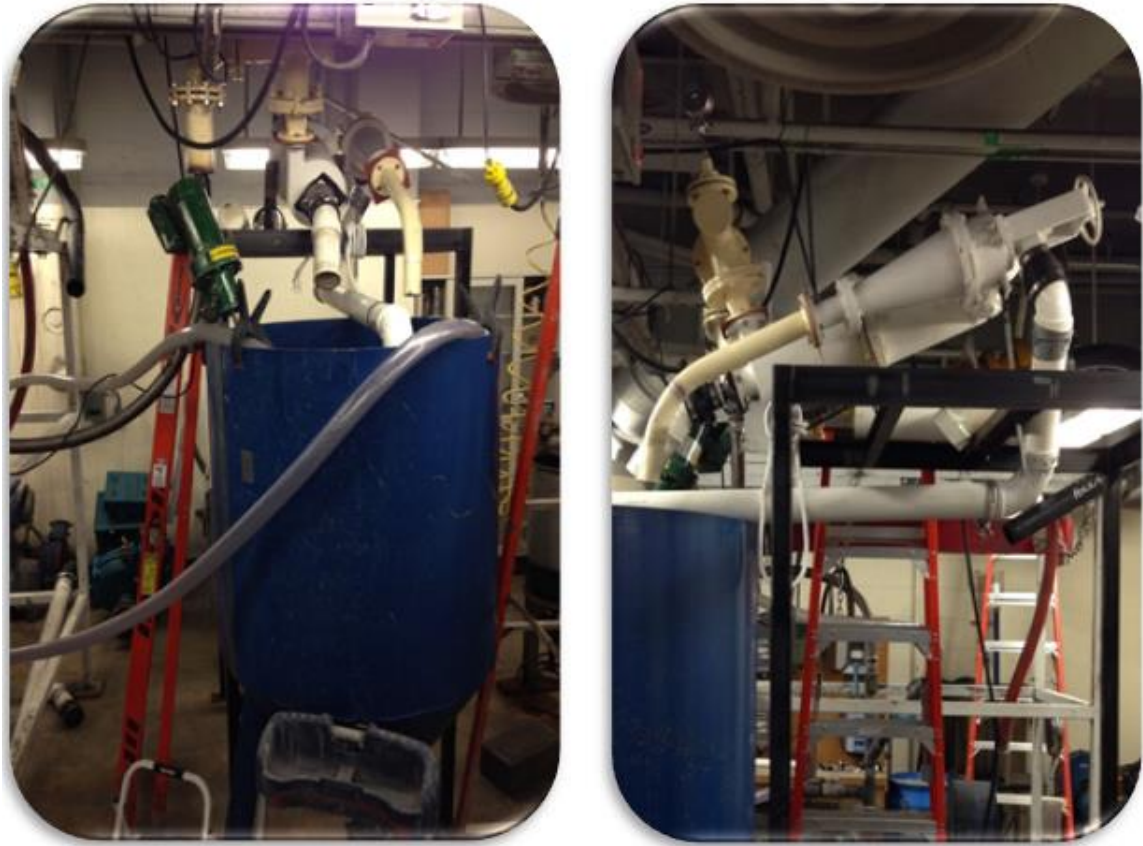
Figure 3.1. GTC three-product DMC circuit with 200-mm (8-inch) cyclone, feed, sump, and pump.
