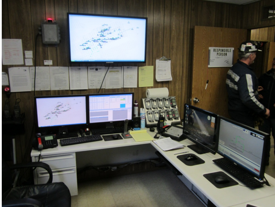
Figure 3-11: Mine Operations Center
