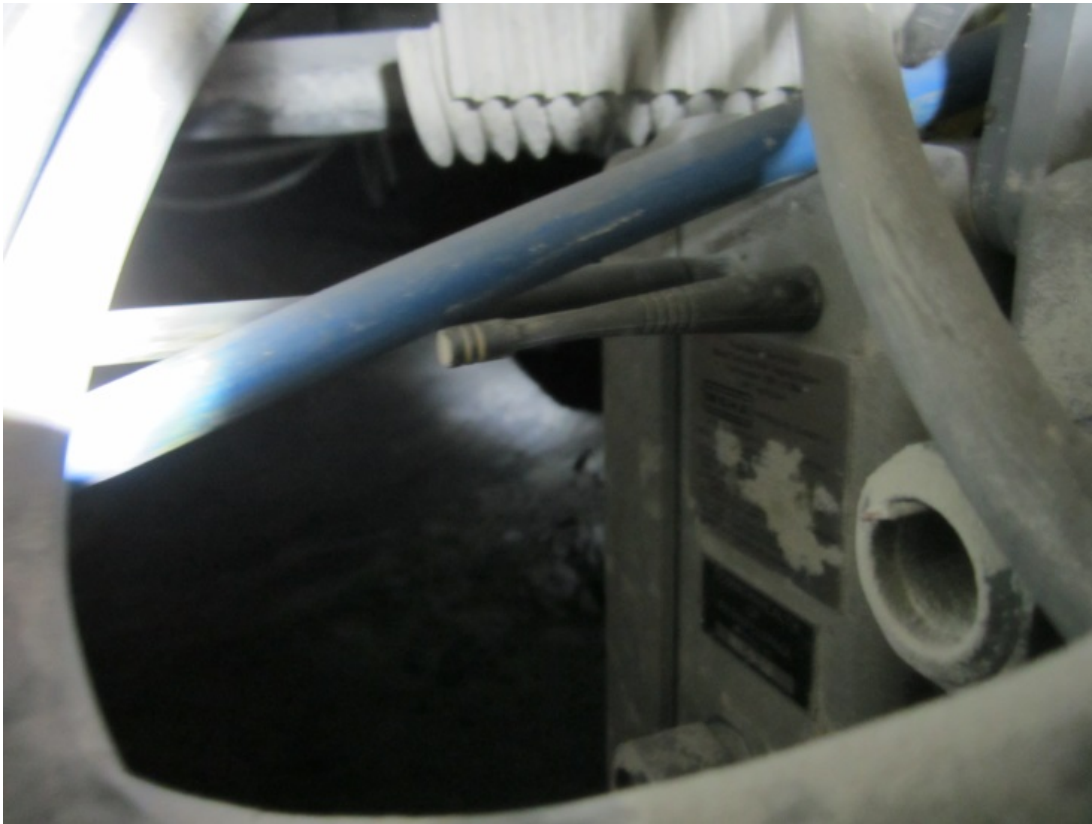
Figure 3-34: Antenna Touching Cable
