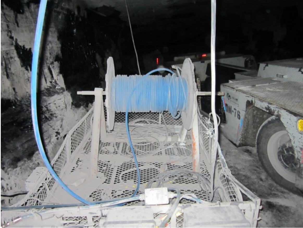
Figure 3-31: Leaky Feeder Cable
