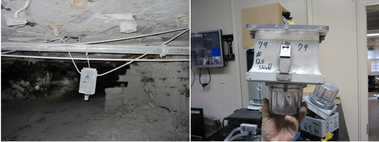
Figure 3-42: Wireless Access Point
