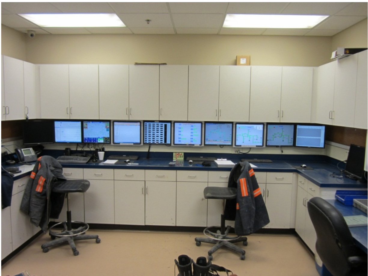
Figure 3-14: Surface Control Center
