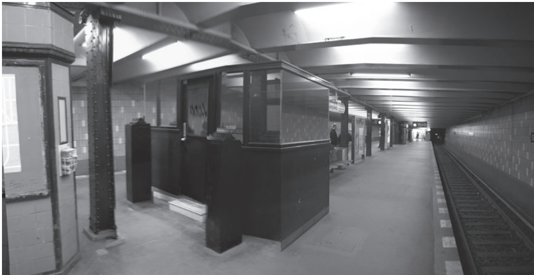
fig 4.01_Switchroom at Senefelderplatz
