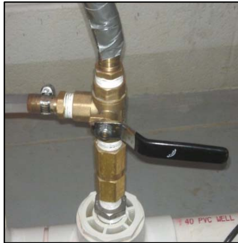
Figure 3.5 Injection line flow control valve
