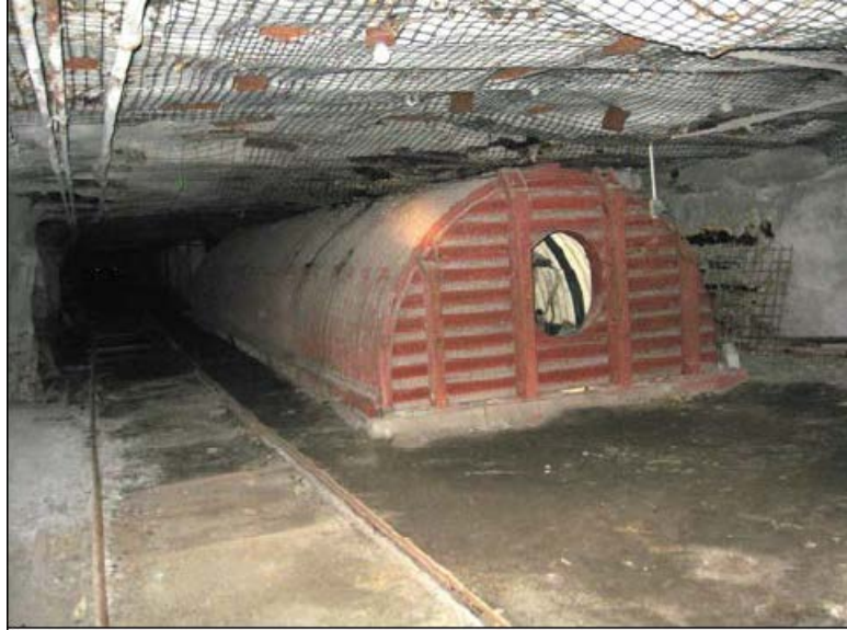
Figure 1.1. Refuge Chamber Located in Bruceton Safety Research Mine (Bauer and Kohler, 2009)
