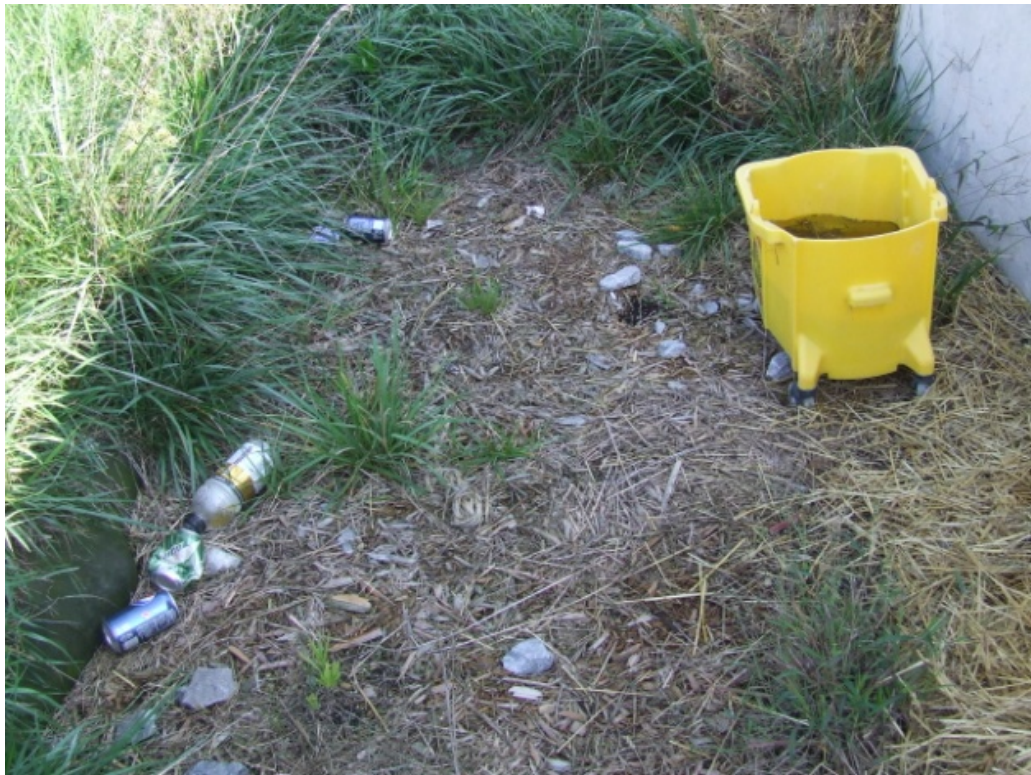
Figure 4.7: Overflow and trash in the rain garden basin at pad X2.
