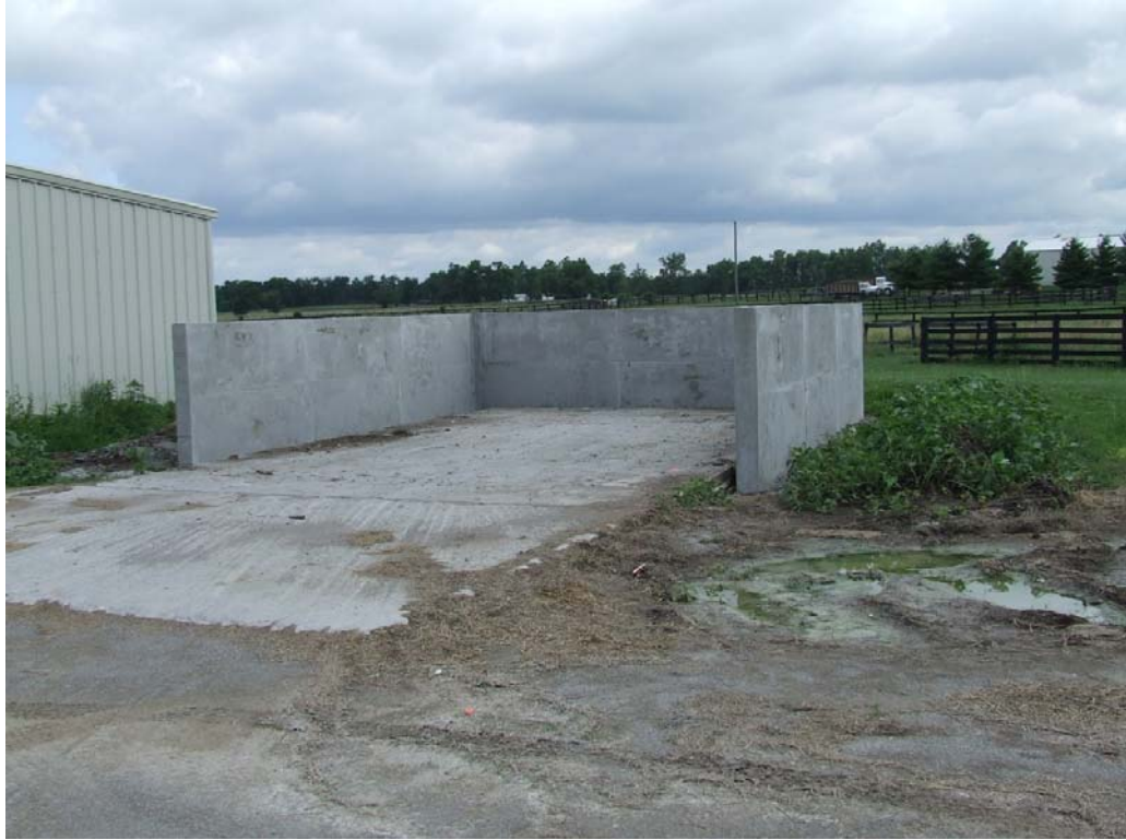
Figure 1.1: Typical muck storage pad at Victory Haven, with concrete pad, walls, and approach.
