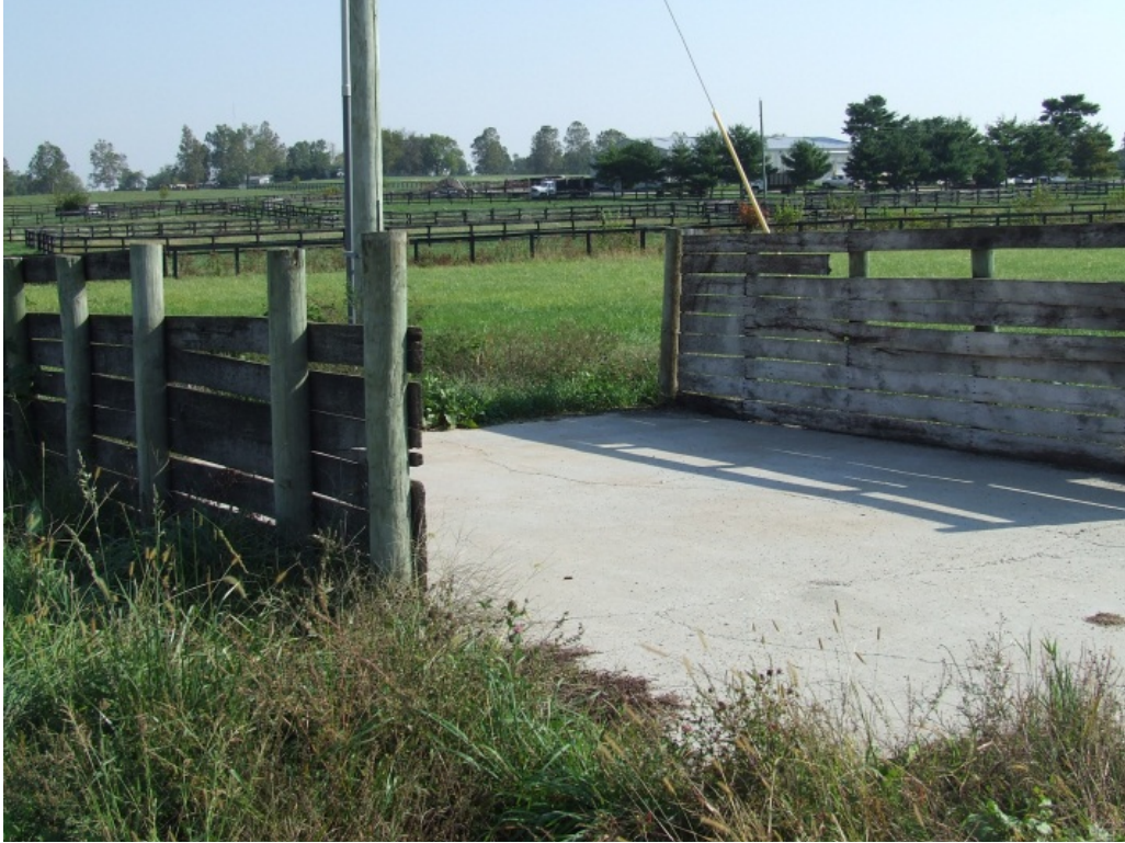
Figure 1.3: Muck storage pad at Victory Haven showing flimsy wooden walls with gaps, allowing for excess spillage and seepage of liquid waste.
