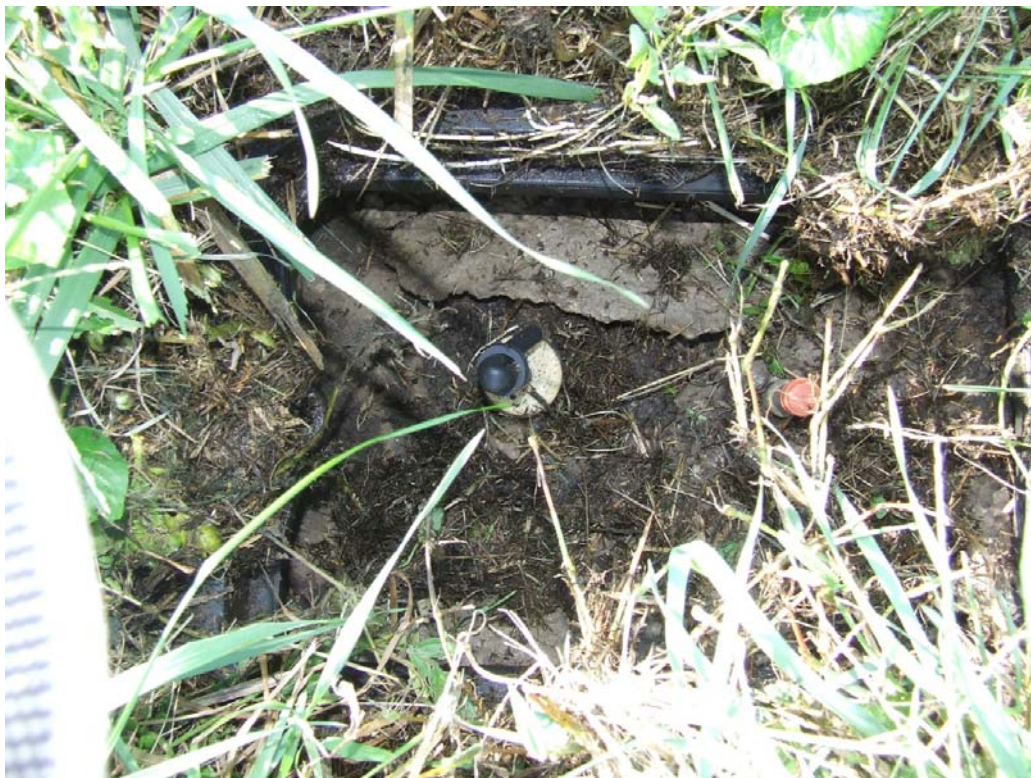
Figure 2.16: Picture of lysimeter and tensiometer in valve box behind pad C1.
