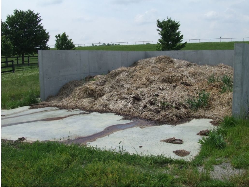
Figure 4.4: Runoff escaping from the approach end of pad X2.
