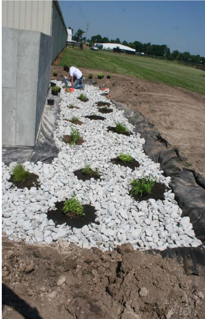
Figure 2.8: Planting of vegetation in rain garden basin at pad X1. Cypress mulch (approximately 4 inches (10 cm) thick) was subsequently placed on top of rock and between plants.
