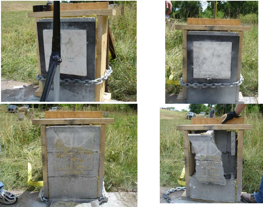
Figure C.3.a, b, c, d Blast 3 - Drywall & Drywall & 16 Ga. Steel (Clock-wise from upper left) (a) C4 charge positioned with tape in front of two layers of drywall and a 16 gage sheet of steel before blast; (b) Condition of foam sample immediately after blast; (c) Front of mock wall after blast and after wall was tilted parallel with ground; (d) Appearance of mock wall after foam sample and steel plate are removed. Some adhesive is visible.
