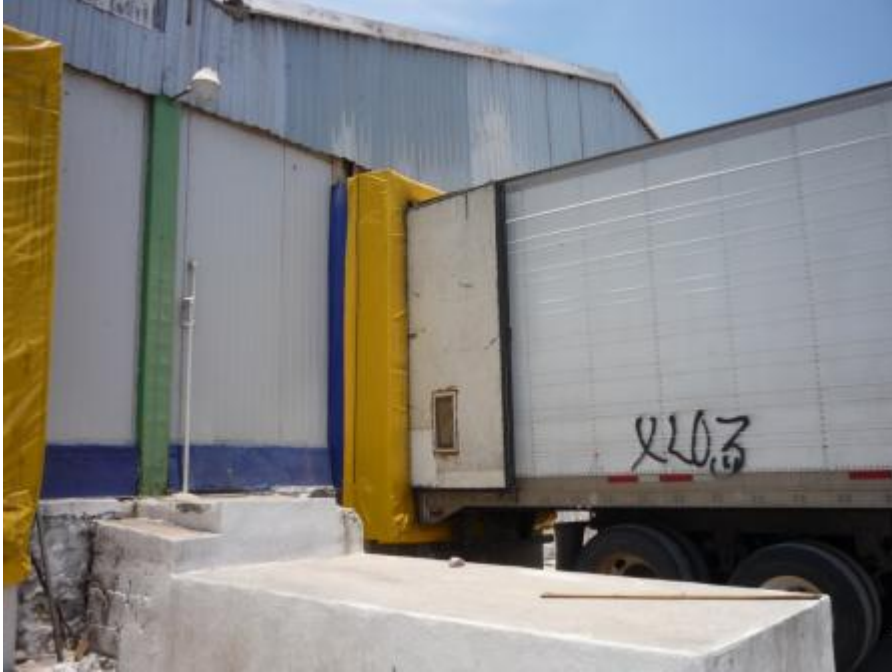
Figure 6-10 A loading dock in a mango packinghouse, Escuinapa, Sinaloa, Mexico. Trailer's rear hatch is tightly pressed against sponge-foams of the dock. (Photo by author)
