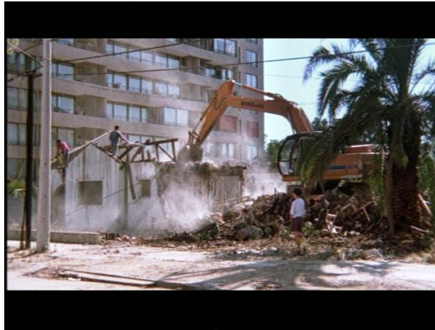
Figure 3.2. The destruction of the house appears both immediate and shocking. Source: Aquí se construye .
