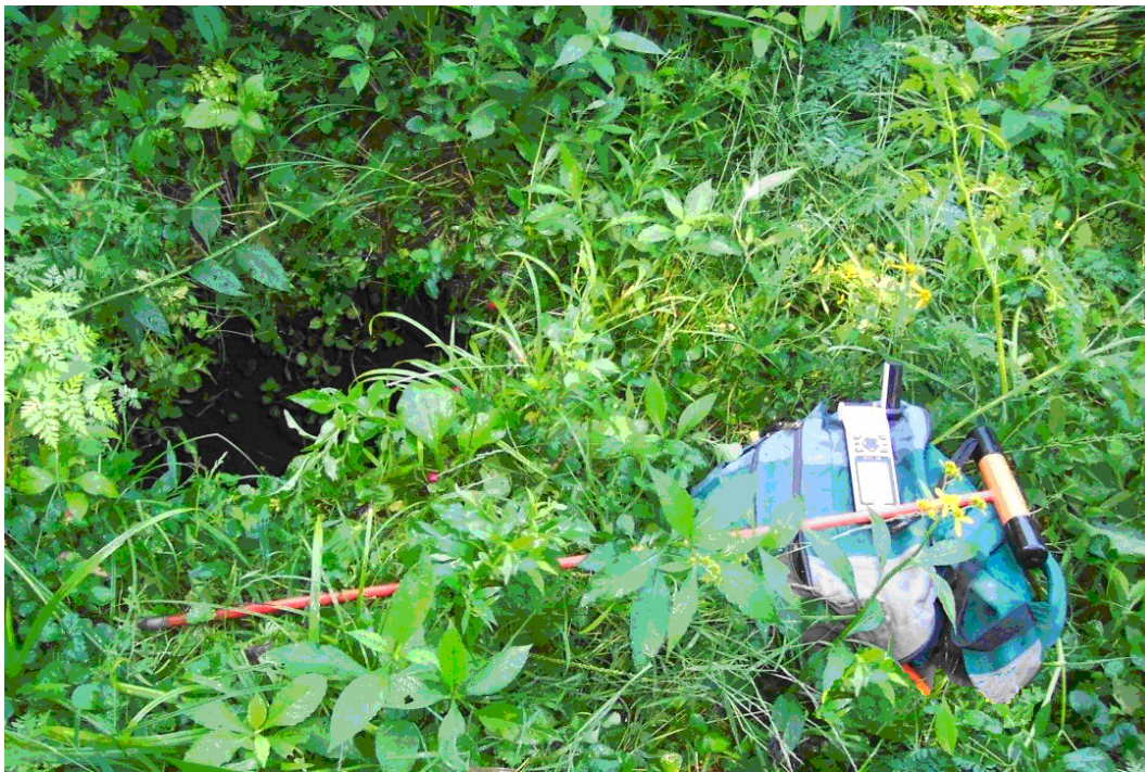
Figure 5.10. Soil cover collapse pit opening revealed on September 18 following a single large rain event the preceding day. Photo by author, September 2004
