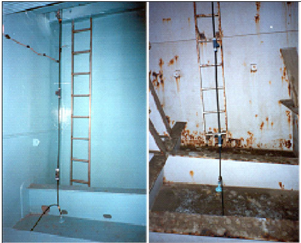
Figure 1.1 Condition of ballast tank after 10 years
