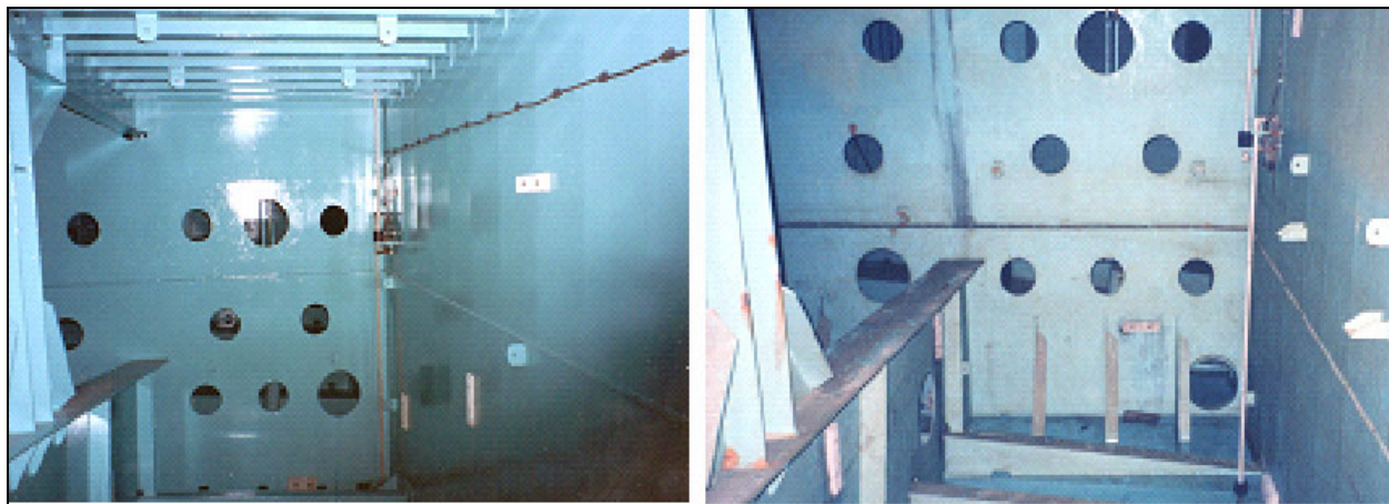
Figure 1.2 Condition of ballast tank after 5 years
