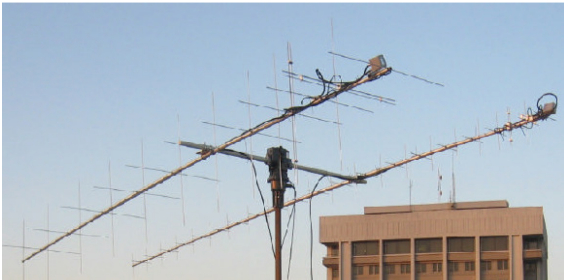
Figure 3.4: A pair of Yagi-Uda antennas at the University of Kentucky used for satellite and amateur-radio communication.
