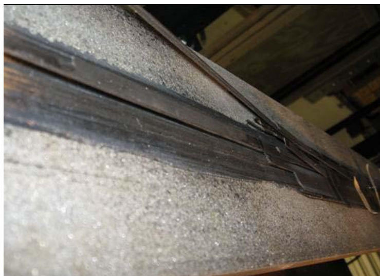
Fig. 2.43: Rupture of full width laminate
