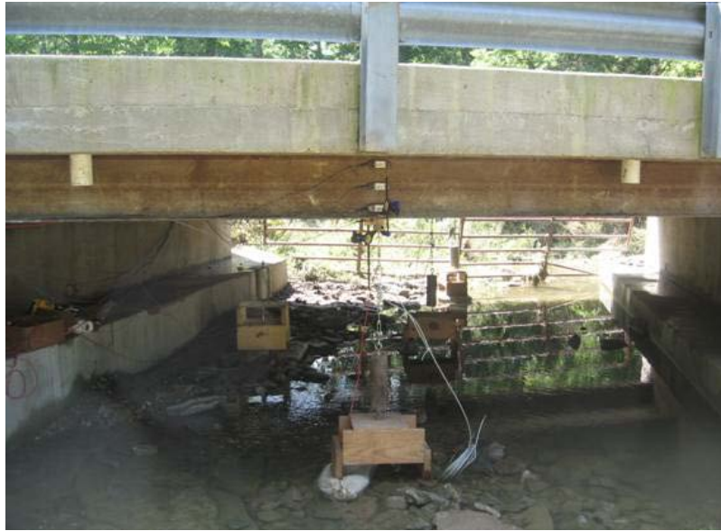
Fig. 5.26: Instrumentation under the bridge at all four locations
