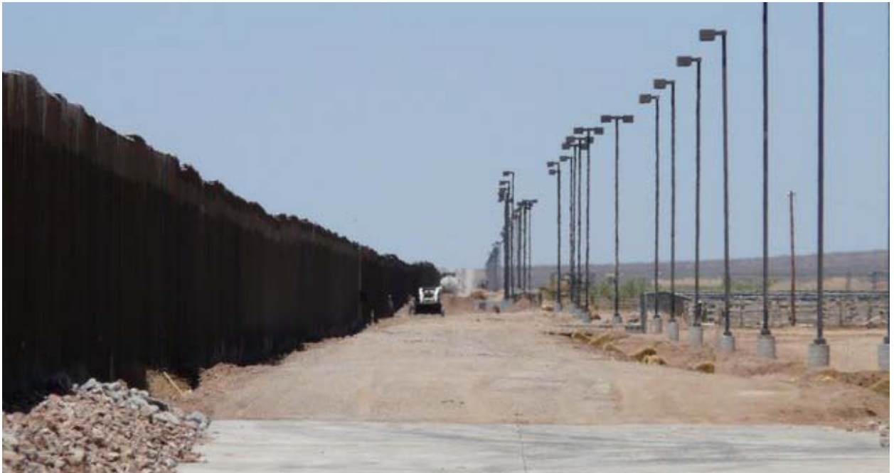
Figure 4.6: Border Fence, Lighting, and Patrol Roads
