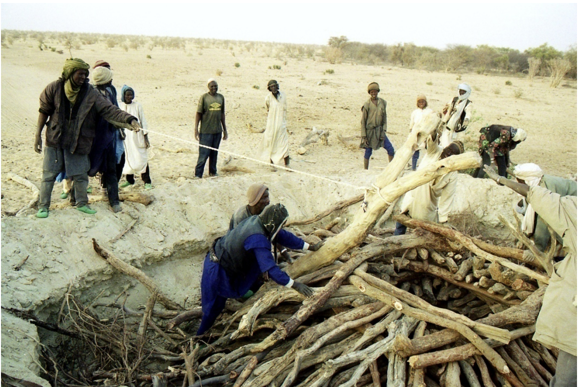
Figure 8.38: (Photo, January 2007) With the new supports in place, the men position the sigitahi.
