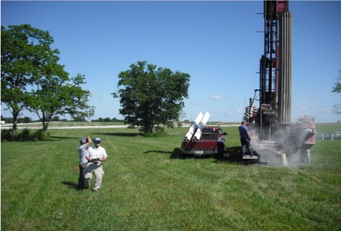
Figure 1.7 Drilling to locate the main karst conduit in the Kentucky Horse Park (photograph taken summer 2008).
