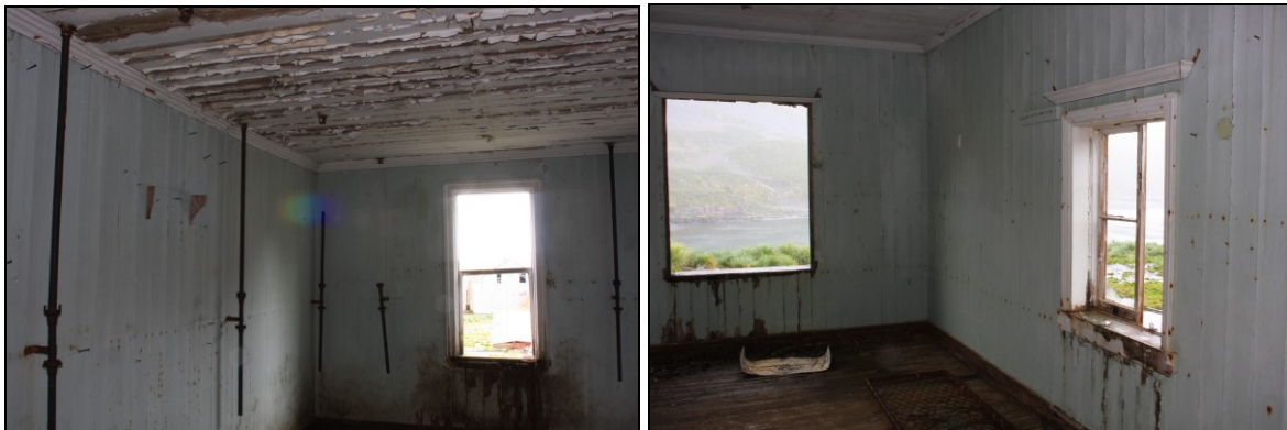
Fig 115 and 116. In barrack 18, eight workers were accommodated in each room. In the eastern part of barrack 19, only two workers shared a room and the standard of these rooms was visibly higher. Photos: Gustav Rossnes. LASHIPA 6/2009.
