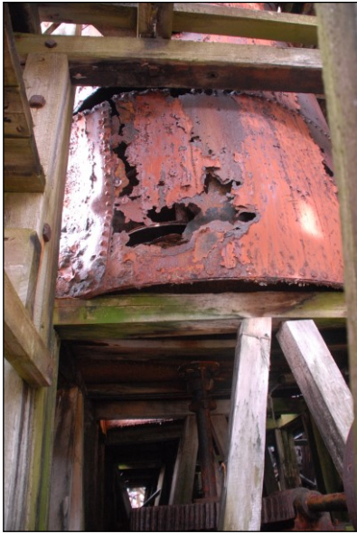
Fig 103. Vertical blubber cooker with rotating mechanism at Prince Olav Harbour in 2009. The internal mechanism is visible underneath and through the rust hole in the cooker. Below is a measured drawing of the blubber cookery where these cookers are located. Photo: U.I. Gustafsson. LASHIPA 6/2009.
