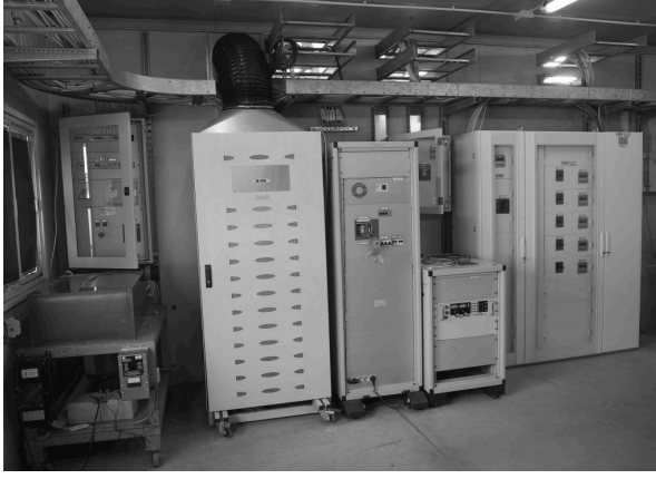
Fig. 2. Photo of the RSE's DC microgrid adopted during the test.
