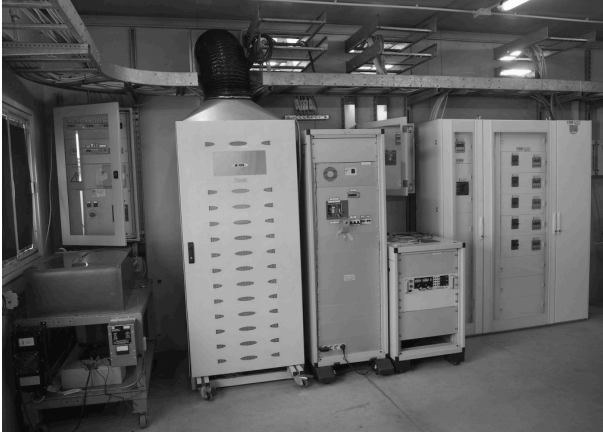
Figure 3. Photo of the RSE's DC microgrid adopted during the test.
