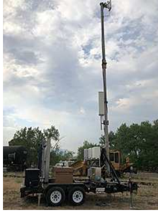
Figure 1.1 Verizon COW used during the 2018 Spring Creek fire in Huerfano County, Colorado. Source: [8].
