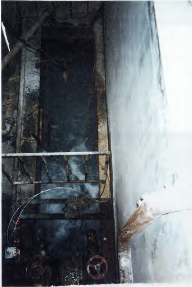
Photograph 7. Discharged Water with High Levels of BOD, COD and SS
