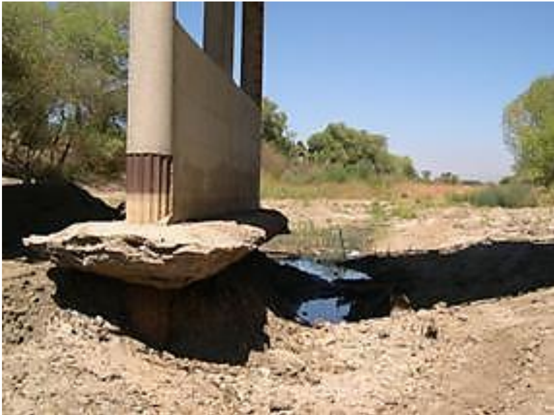
Figure 1.1 Pier scour, Murietta Creek, Pacific Coastal, (FHWA 2006).
