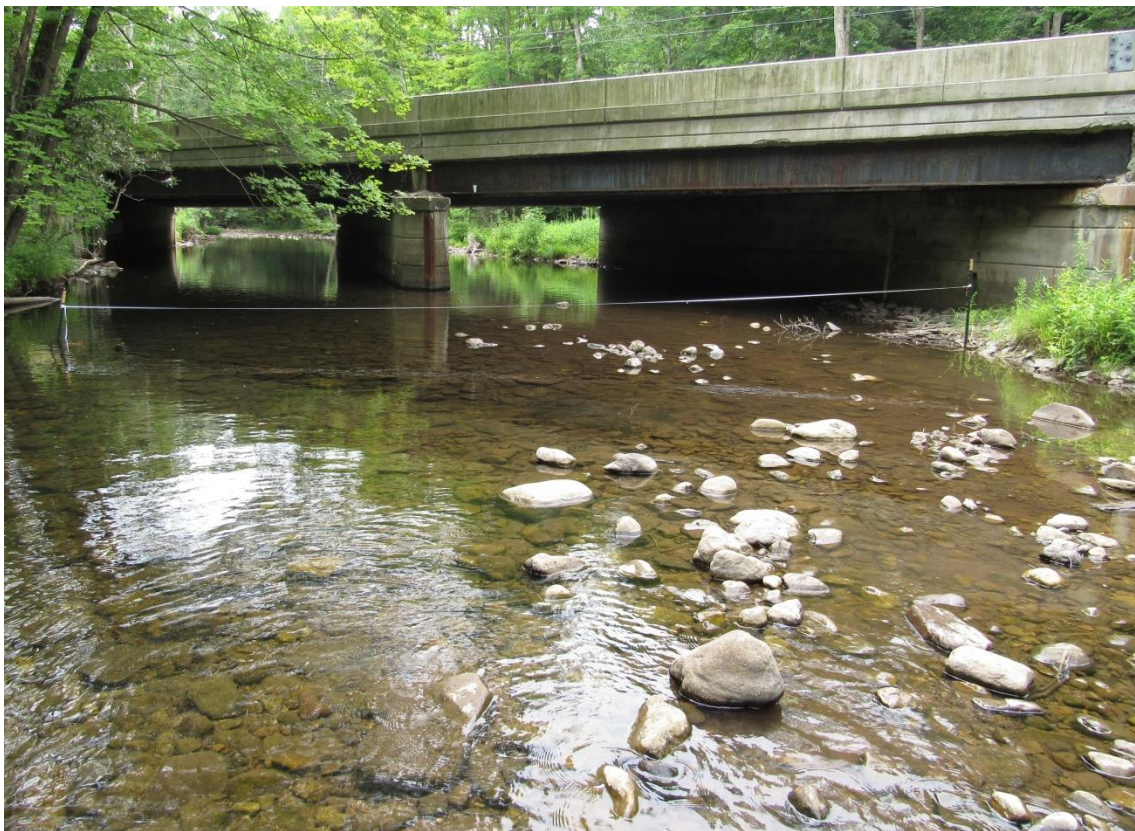
Figure E.28 Bridge # 1912-160 elevation, up-stream looking down-stream, and Wolman Pebble Count section installation.
