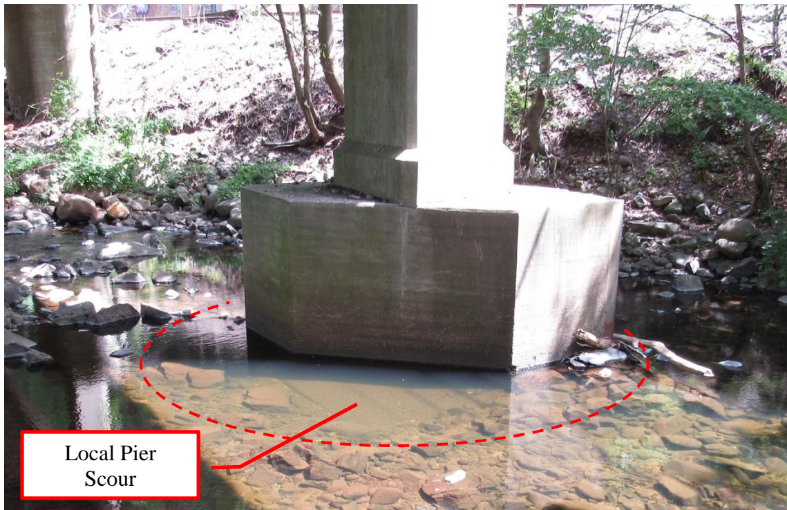
Figure 2.7 Local scour at a pier, bridge # 1405-156.
