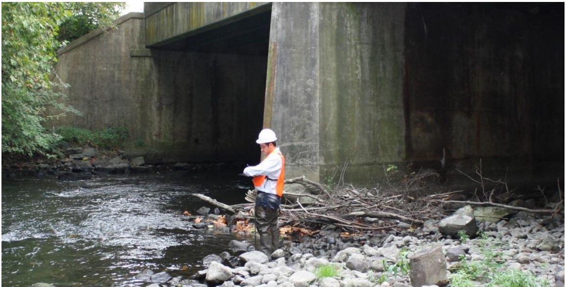
Figure 2.5 Debris build-up in the waterway, bridge # 2107-156.
