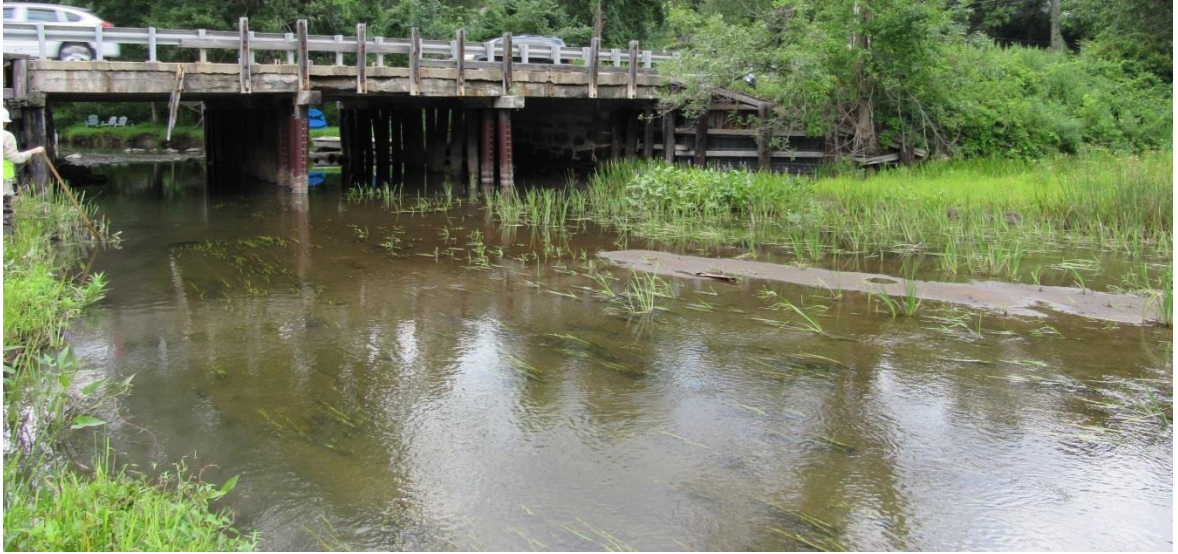
Figure 2.4 Contraction scour, bridge # 1404-158.
