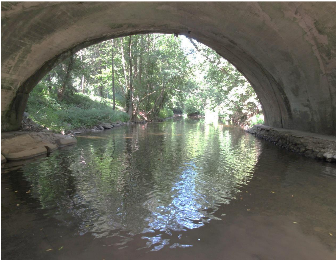
Figure 2.2 Streambed long term degradation, bridge # 2103-152.
