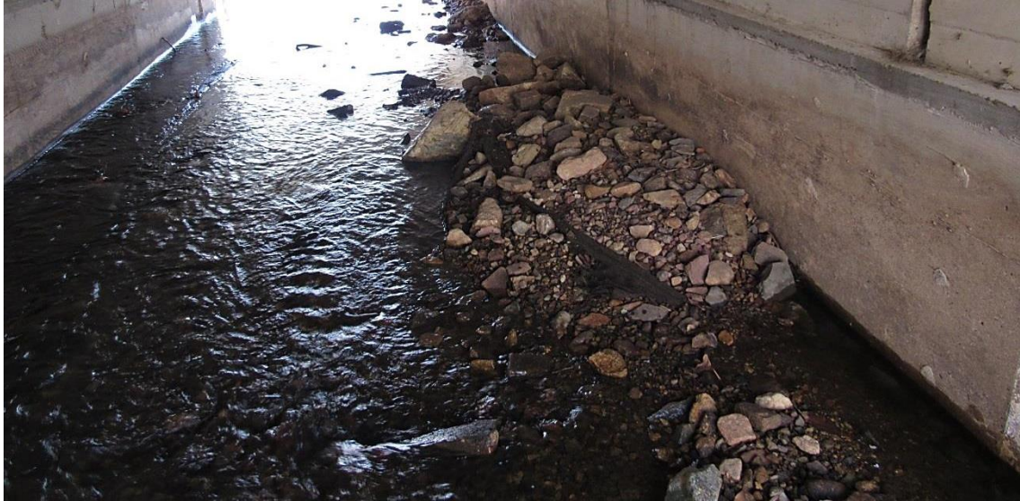
Figure 2.1 Streambed long term aggradation, bridge # 1809-153.
