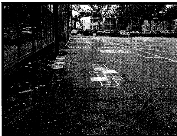
I.2 Water drainage is problematic after a rainfall.
