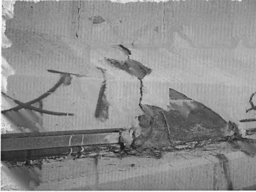
Figure 2.16 Diaphragm crack at fascia beam (Rt. 1&9, Newark).
