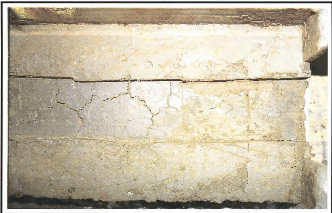
Photograph A-16. Note that the wetting also caused the vertical shrinkage cracks to seal at the fracture level.
