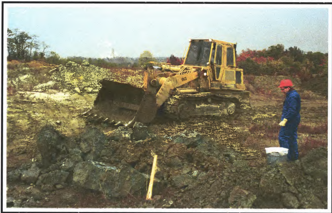
Photograph A-3. The Potomac Formation clays required excavation by a bulldozer. The blue and red clays are shown to the left and right, respectively.
