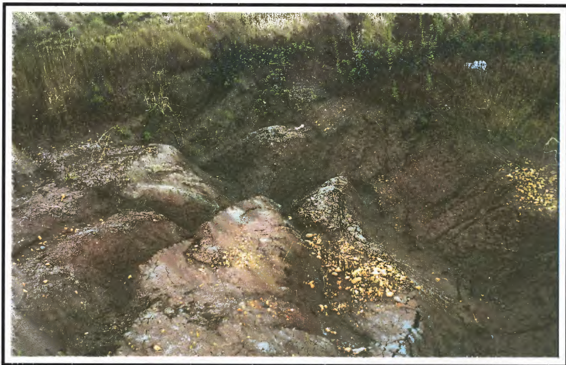
Photograph A-1. Gullies formed by erosion of weathered, unvegetated Potomac Formation clay, Rainwater Landfill, Lorton, VA.
