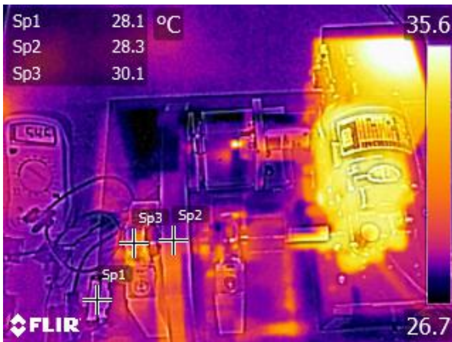
Figure 5.6 Thermal image of the charging system for charging for 20 minutes.
