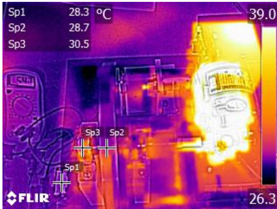
Figure 5.7 Thermal image of the charging system for charging for 30 minutes.
