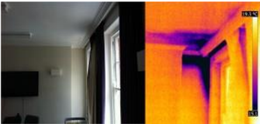
Figure 4.4 Infrared imaging of damage in wall due to moisture.
