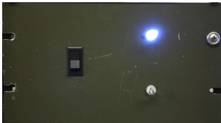
Figure 5.22 TPGV Control Panel.
