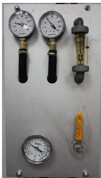
Figure 5.9 GXS Water Flow Control Panel.
