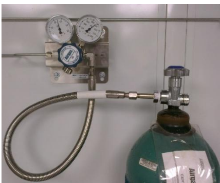
Figure 5.35 Gas Regulator and Flexible Hose (Attached to the Gas Cylinder).
