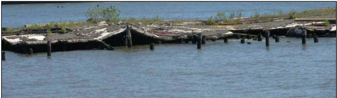
Figure 6.7 Rotted pier in the Hudson River, Hoboken. 2011. Personal photograph by author. This pier was once used for the transference of cargo from ships on the Hudson River to the shores of Hoboken, New Jersey.
