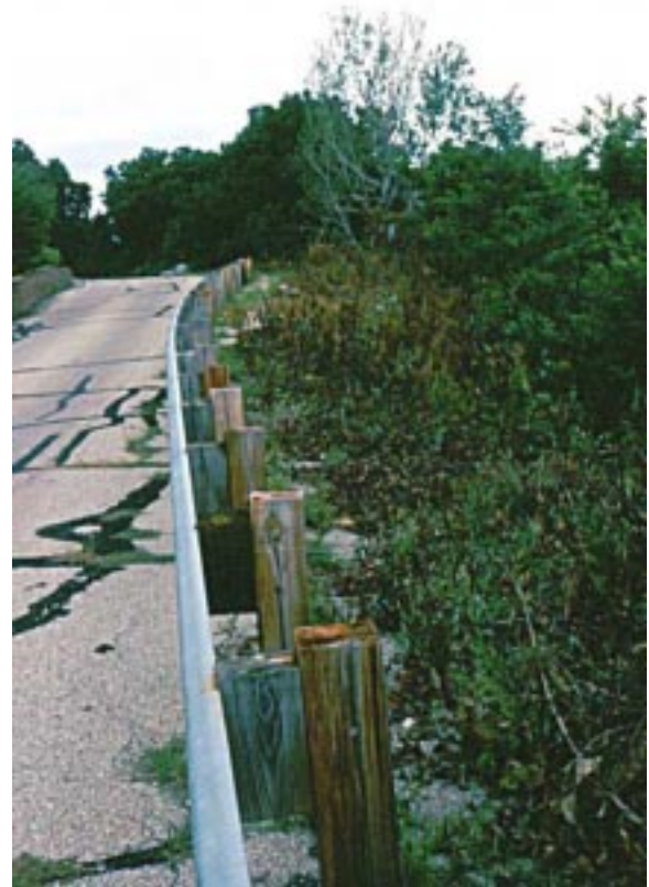
FIGURE 9. Scarp of the recent landslide along Riverview Drive (see fig. 8). The landslide has removed one lane from the street.
