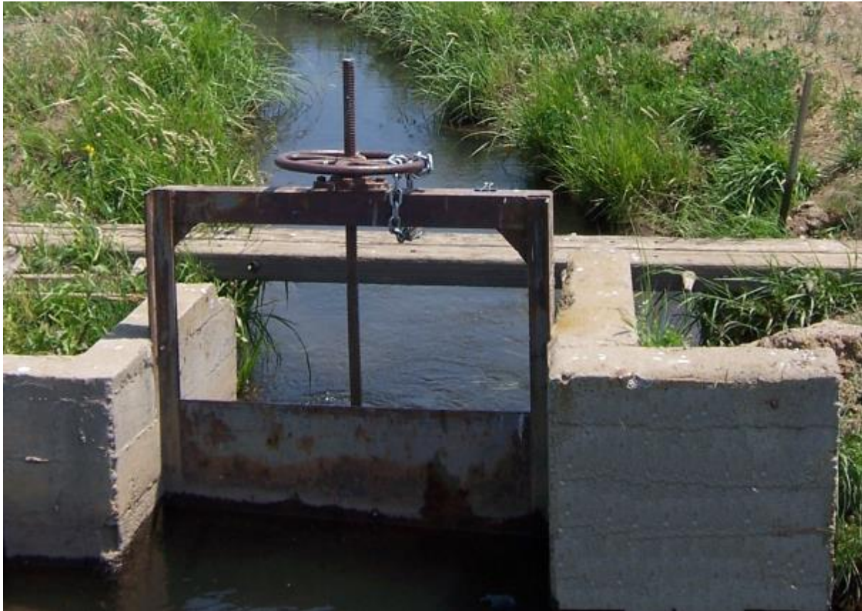
Figure 4-1 Example of a Flow Diversion Gate (Accessed 5/07/2019 from https://medium.com/@ShawnH2O/can-i-lose-my-california-water-right-7ea825226831 )
