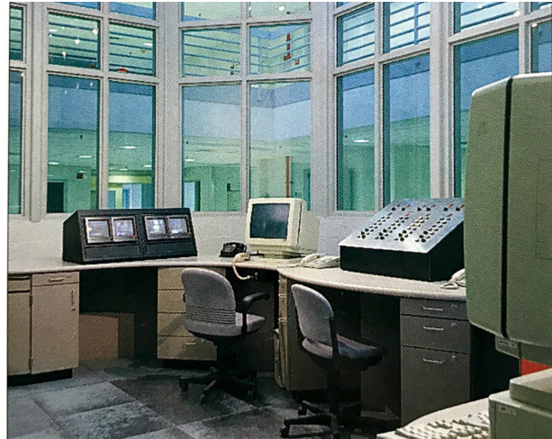
Figure 02-03-06. Control room in Leon County Detention Facility, Florida, USA
