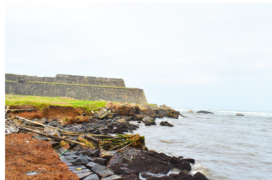
Figure 6: Effect of sea erosion at Galle Fort (Photo credit: Amila Bandaranayake)
