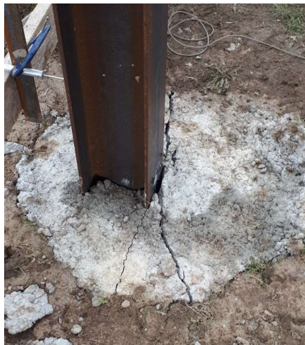
Figure 4-4: Crack in DS-02 during lateral load test.
