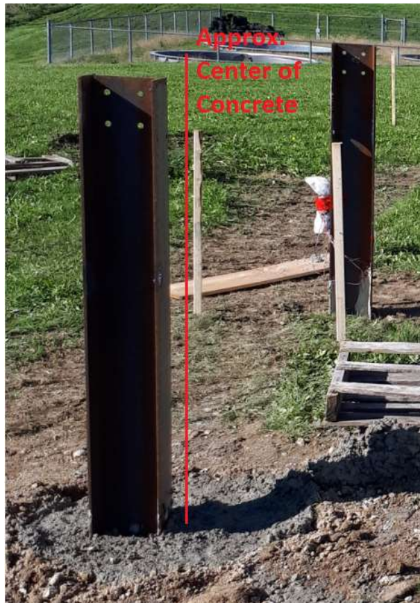
Figure 3-9: Misaligned reinforcement for DS-02.
