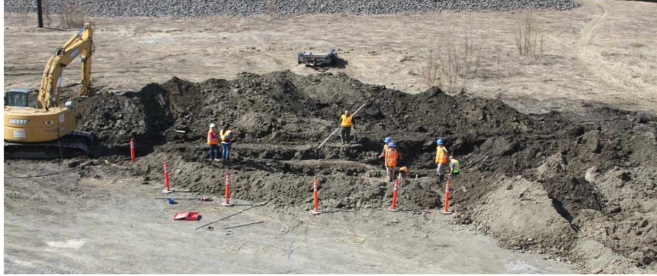
Figure 2.3. GHE slinky coil installation. The installation of the GHE required a large excavation that took nine days.
