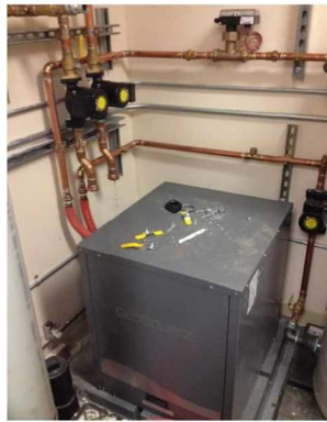
Figure 2.4. Heat pump and plumbing installation. The heat pump plumbing involved setting the heat pump and the buffer tanks and connecting all the parts with copper pipe.
