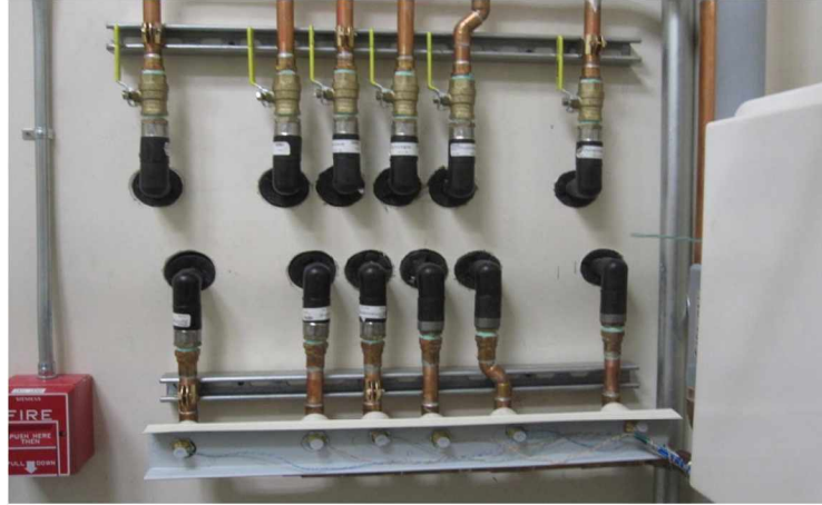
Figure 2.7. GSHP manifold. The manifold is located in the mechanical room. Temperature sensors are in thermowells on the return loop from the ground side of the GHE (the bottom in this photo).
