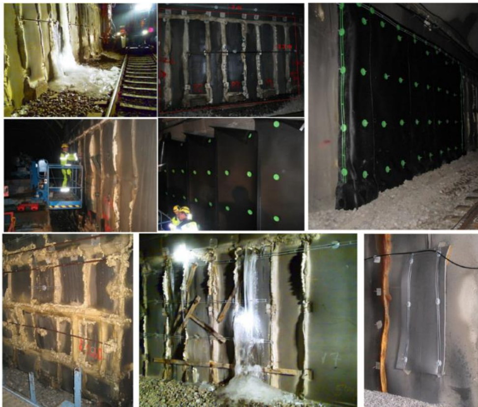
Figure 2.33: The local maintenance performed on the frozen section of the tunnel lining by installation of the new membrane, Finland [140].
