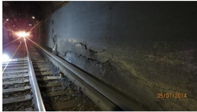
Figure 2.11: Damages on Amtrak's 104-year old Hudson River tunnels, New York, the USA [38].
