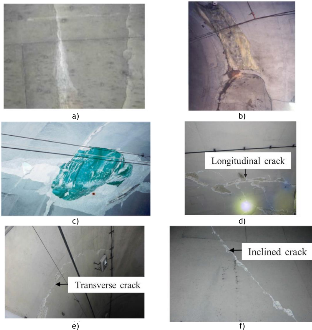
Figure 2.1: Typical cracking defect examples in concrete: a) crack with efflorescence [26], b) spalling of lining extended to the opening [27], c) crown spalling [27], d) longitudinal cracks of crown [28], e) transverse crack [28] and f) inclined cracks of side wall [28].
