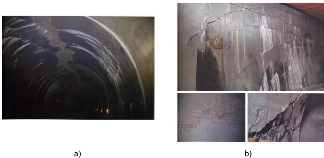
Figure 2.8: a) Spalling and dense cracking of the liner inside the Longxi tunnel and b) inclined cracking at the sidewall with water leakage and spalling [35].
