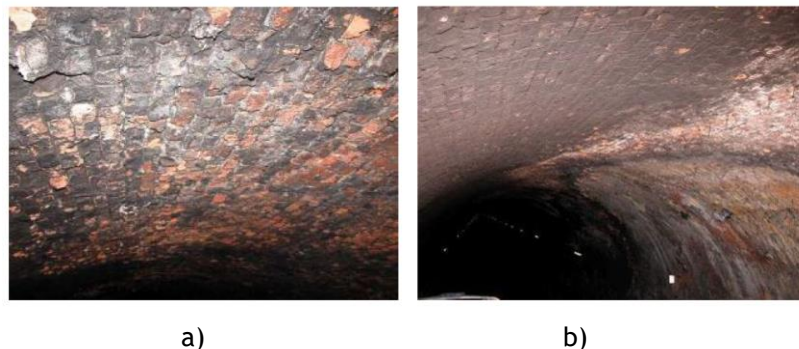
Figure 2.13: Damage on Rossio Railway Tunnel; a) deformation and erosion of the masonry on the vault surface and b) deformation on vault section [39].
