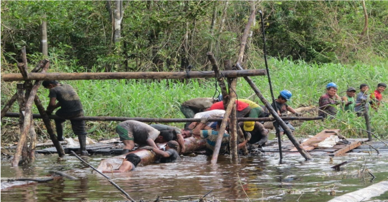
Photograph 7.4: Cocama work without protective clothing locating the pipeline break.
