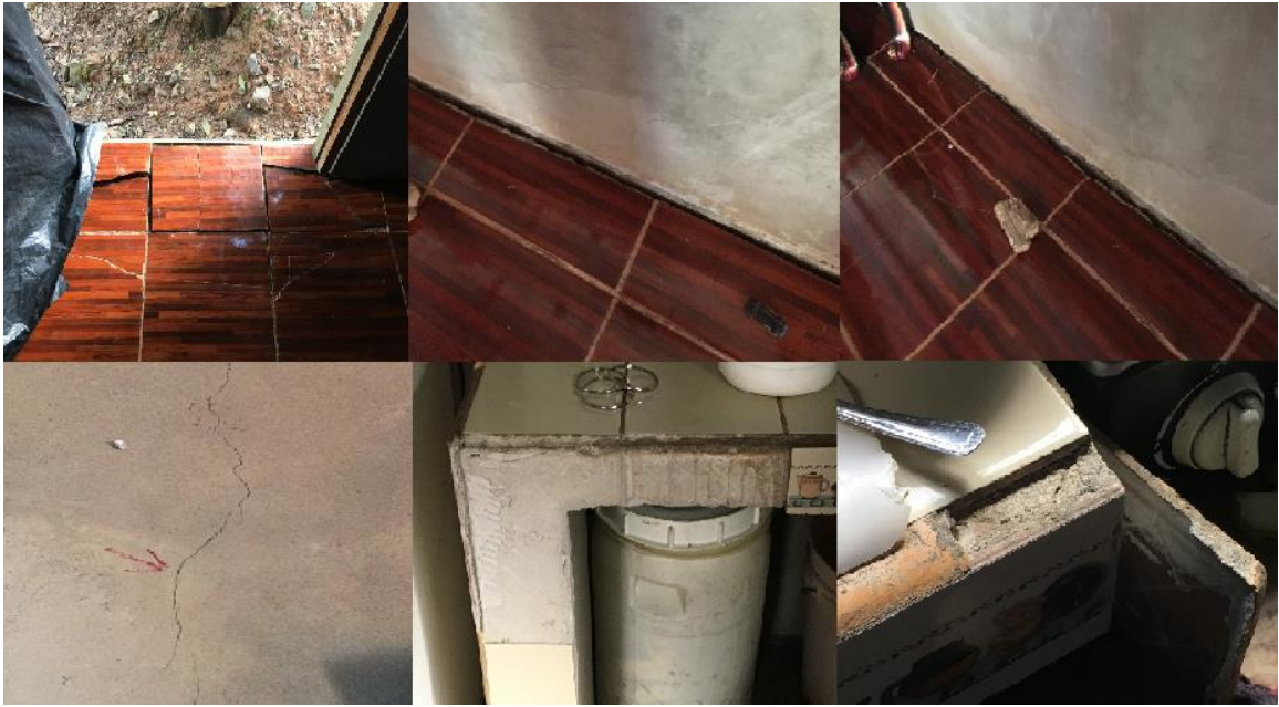
Figure 6.2A: Destruction of Homes by B2Gold's Explosives
