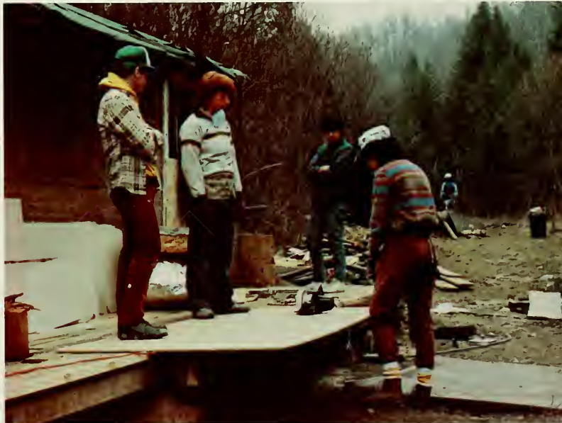
Rebecca Efrogmson has many supervisors as she prepares to cut a piece of "sheetrock."
