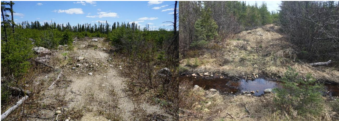
Figure 7. Examples of reclamation techniques. Left, scalloping of the roadbed with aggregates and coarse woody debris. Right, a water-crossing removal at a road entrance from an active road segment creating a channel or trench. The culvert removal also acts to potentially bar vehicle access.
