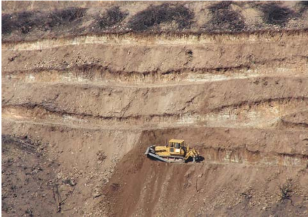
Fig. 1. Illustration of terrace construction, using a bulldozer, on a very steep slope in a recently burnt area in central Portugal, in preparation of new Eucalypt plantation.
