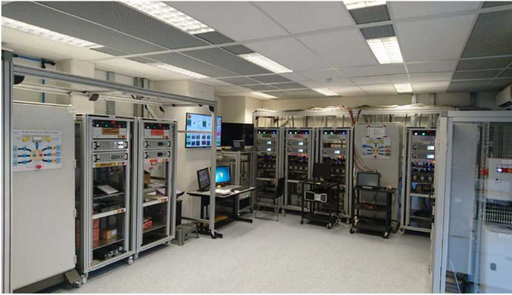
Fig. 7. LAPLACE Lab facilities: smart microgrids investigation testbench.
