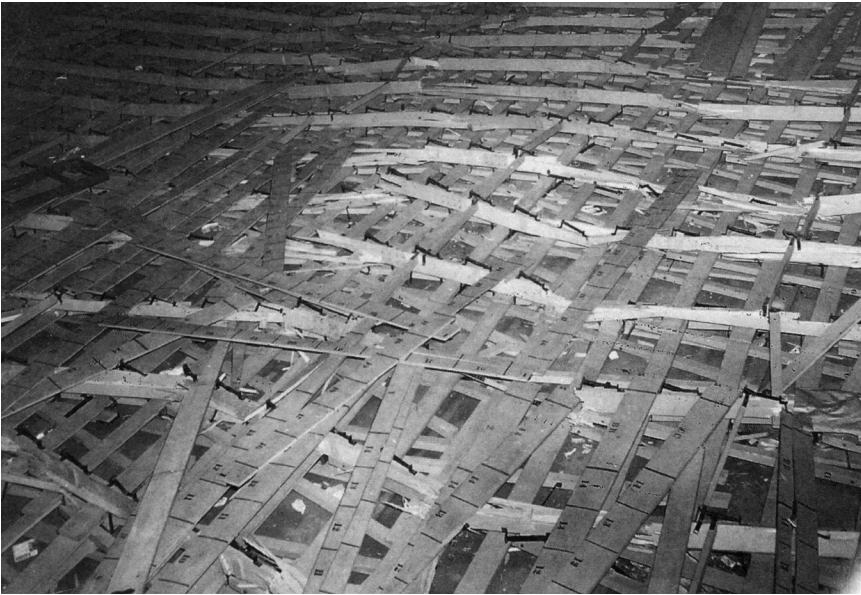
COLLAPSED BLEACHERS. “It was like riding a roller coaster down,” one student said, when the bleachers collapsed during a Purdue basketball game in 1946.
