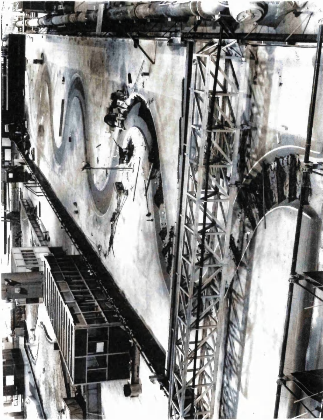
Fig (3.19) - Phase of Construction of The S.E.R.C. Flume Series B with Sinuosity 1.374 and Trapezoidal Cross-Section.
