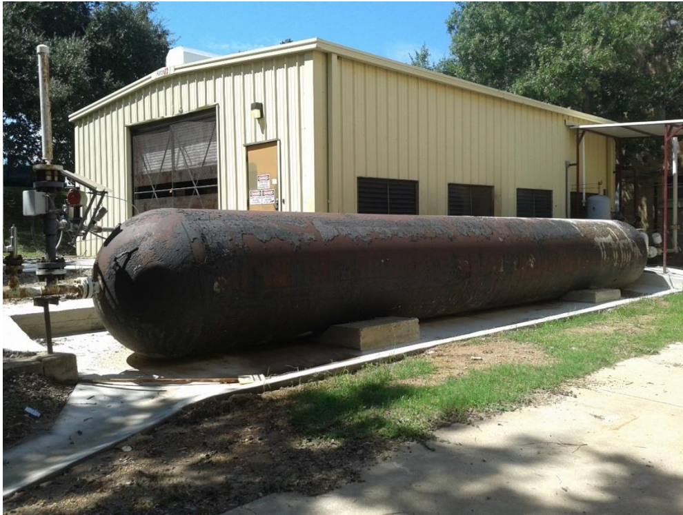
Figure 44. Air storage tank
