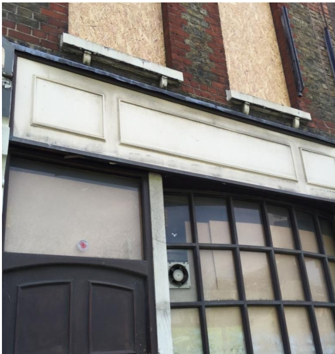
Figure Twenty Three: Boarded up building, Chiswell Street
